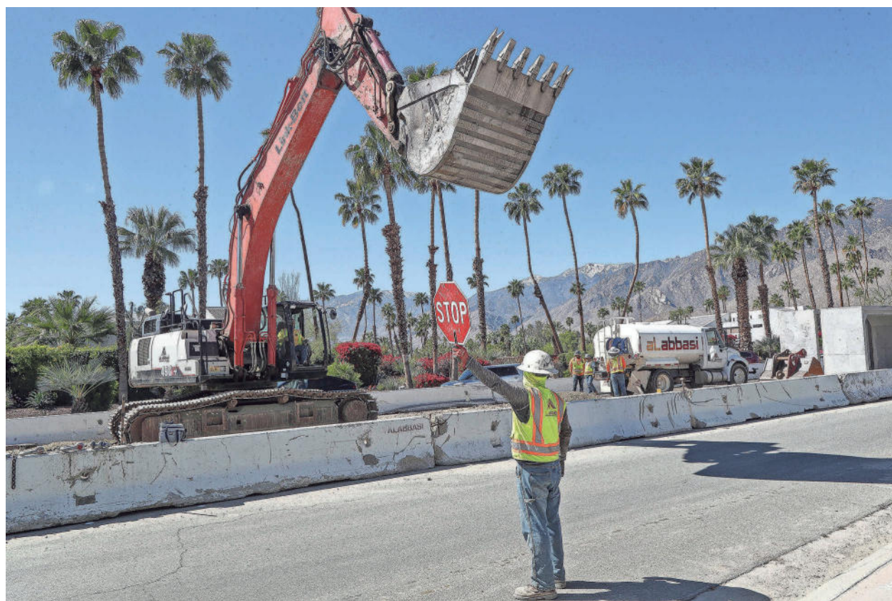
Construction workers construct a major storm drain and flood control line on Ramon Road near the intersection of Compadre Road in Palm Springs on Wednesday. PHOTOS BY JAY CALDERON/THE DESERT SUN
