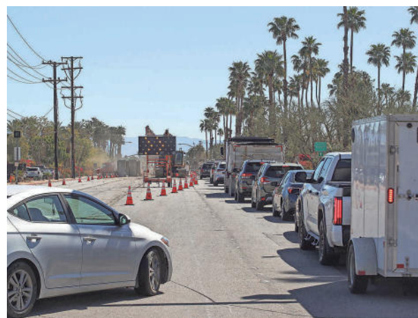
Vehicles merge last week into one lane on eastbound Ramon Road. The work zone will gradually move west along Ramon Road to Farrell Drive and then north on Farrell Drive to Tahquitz Canyon Way.
